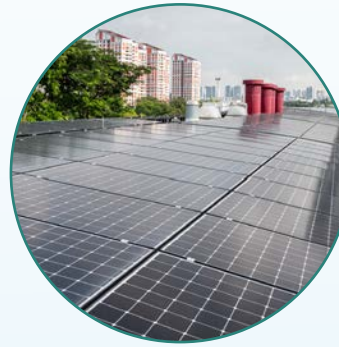
High Efficiency Solar PV System
